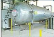
CO2 OPERATION, CO2 TANK AND BOTTLE FILLING
